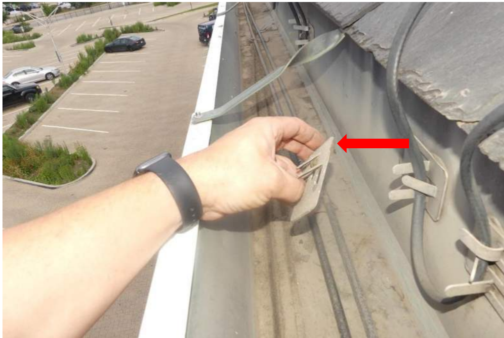
Photo 8 – At 2 locations, clips had become displaced from the gutter.
