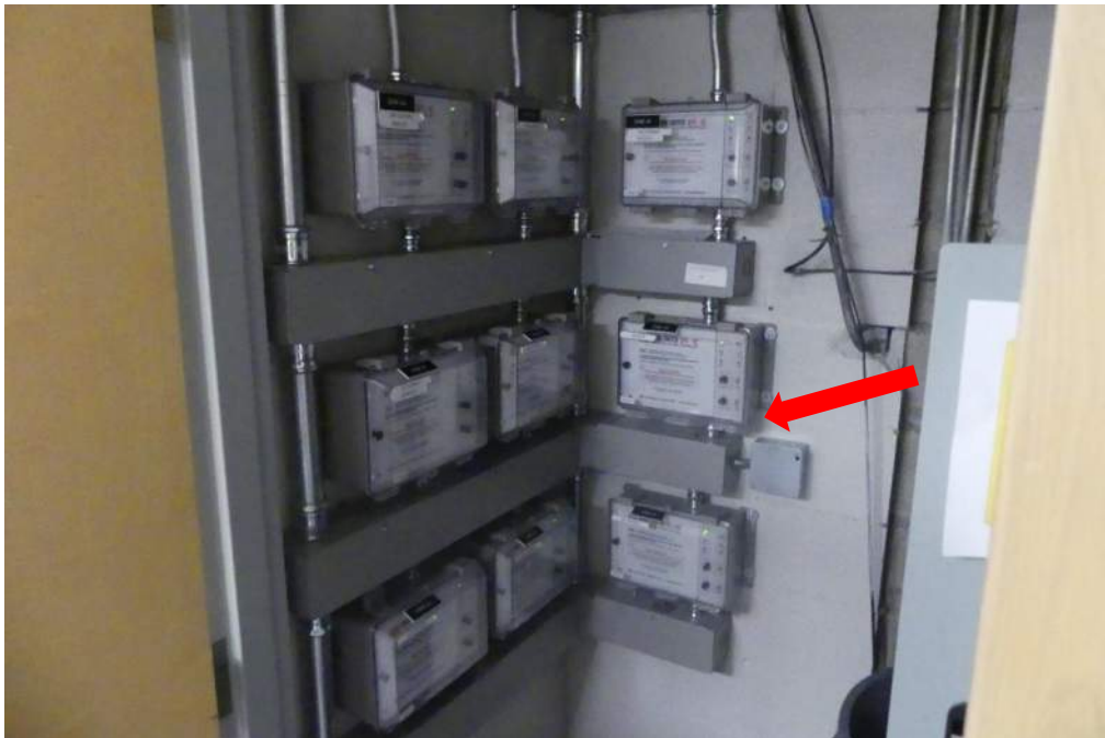
Photo 22 – The controllers were monitored from the building interior.
