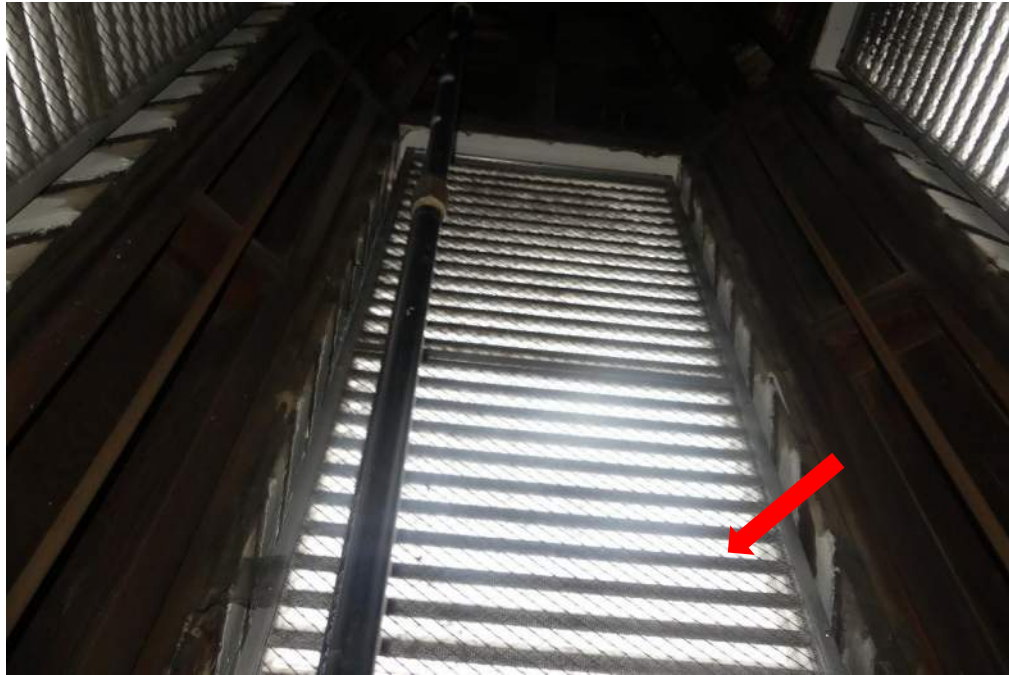
Photo 19 – Within the attic, ventilation was observed to be achieved via a vented cupola at the southeast corner of the roof.
