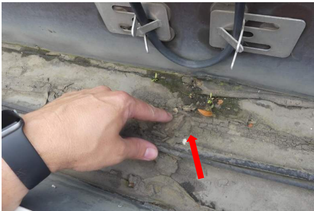
Photo 14 – Along the west gutter and at the north gutter, dirt build-up was observed in the gutter, suggesting that the gutter may not have sufficient slope at these locations.
