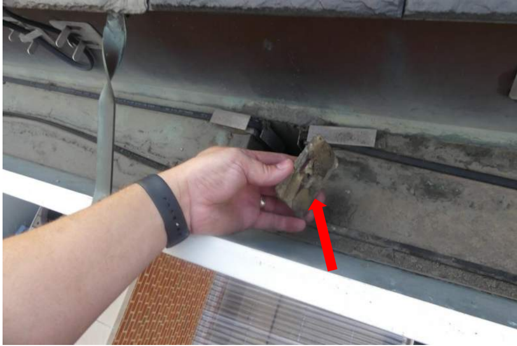
Photo 9 – At 2 locations, clips had become displaced from the gutter.
