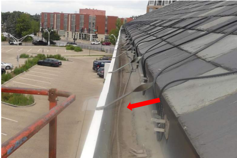
Photo 13 – Along the west gutter and at the north gutter, dirt build-up was observed in the gutter, suggesting that the gutter may not have sufficient slope at these locations.
