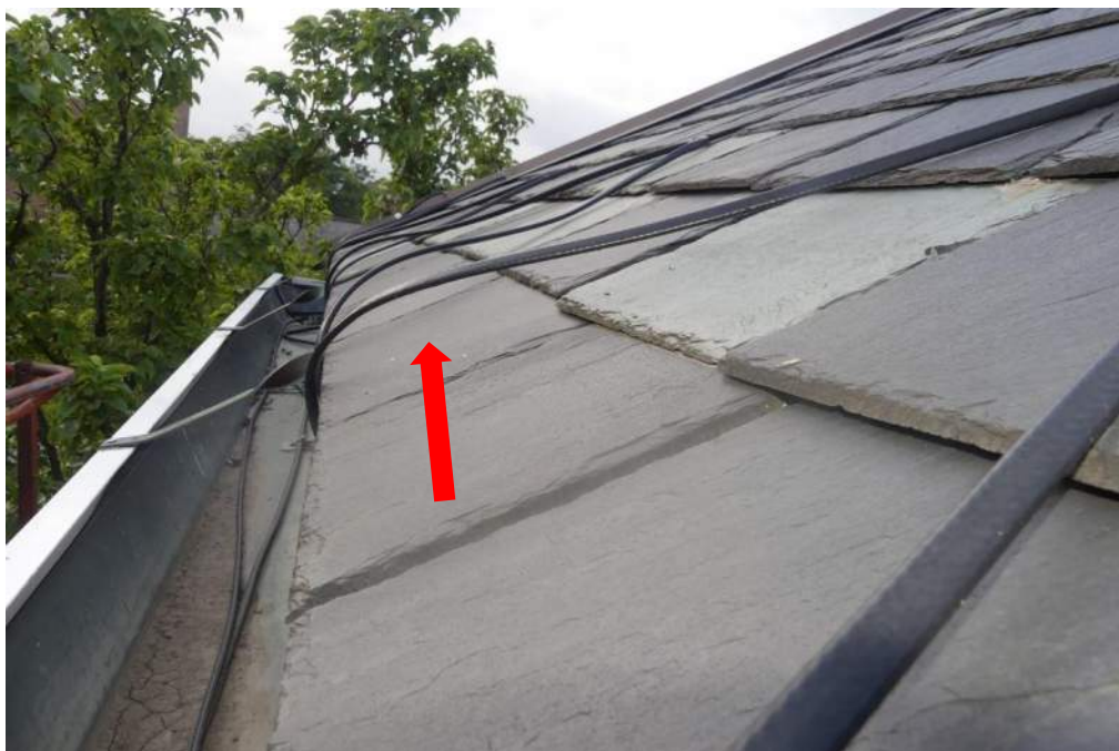
Photo 12 – In some locations, the cables did not make contact with the slate surfaces immediately above the gutters.
