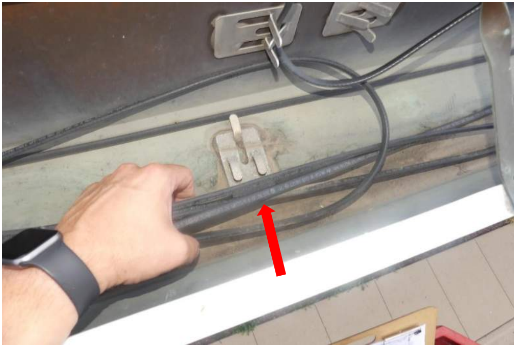
Photo 10 – At the north end of the west gutter, several cables looped in the gutter and were not secured.
