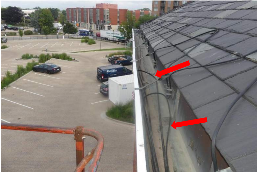
Photo 11 – At the north end of the west gutter, several cables looped in the gutter and were not secured.
