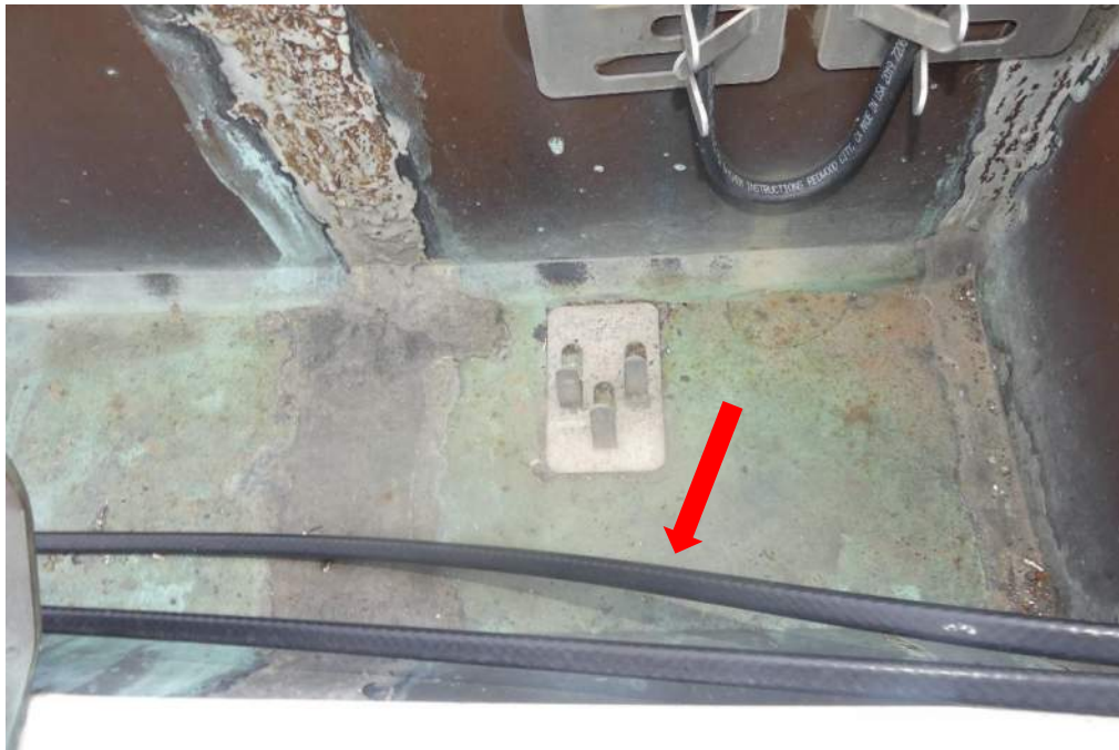
Photo 4 – At several locations, the cables had become displaced from the clips.
