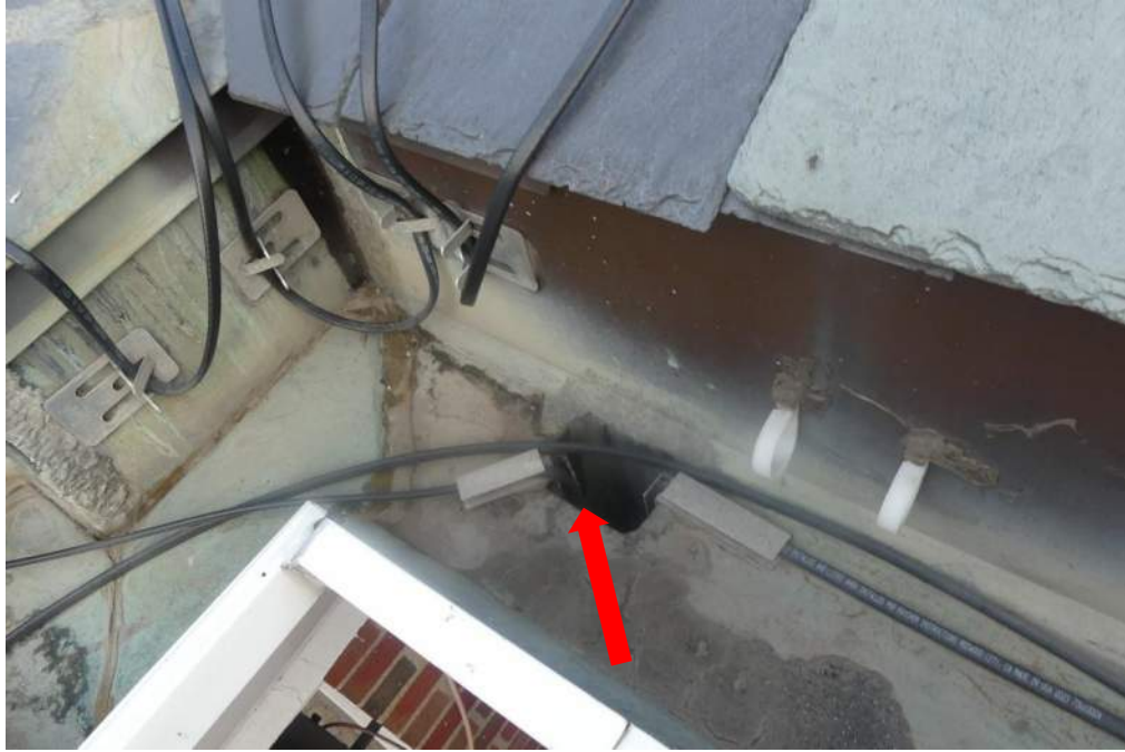
Photo 3 – The cables also extended into the downspouts.
