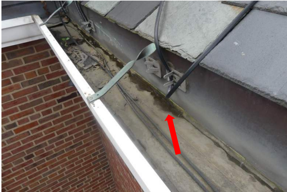
Photo 15 – Along the west gutter and at the north gutter, dirt build-up was observed in the gutter, suggesting that the gutter may not have sufficient slope at these locations.
