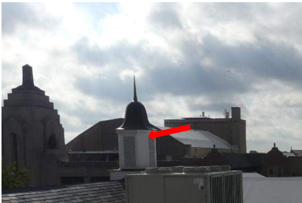
Photo 18 – Within the attic, ventilation was observed to be achieved via a vented cupola at the southeast corner of the roof.
