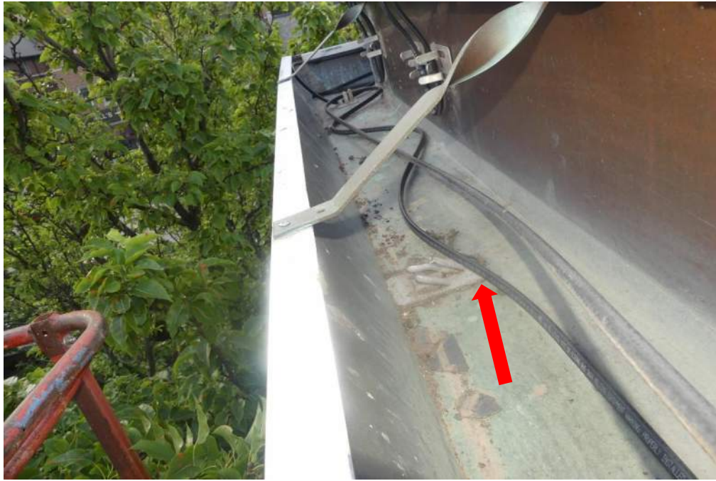
Photo 5 – At several locations, the cables had become displaced from the clips.
