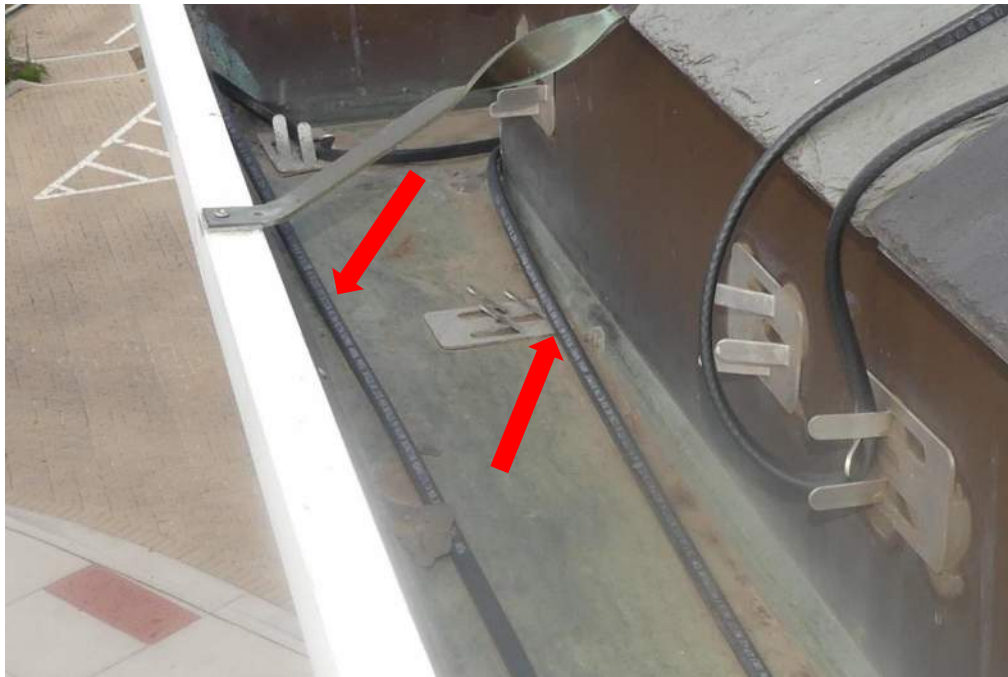
Photo 6 – At several locations, the cables had become displaced from the clips.
