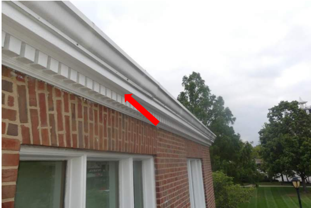
Photo 17 – Along the eaves of the mansard roofs, no ventilation was observed.
