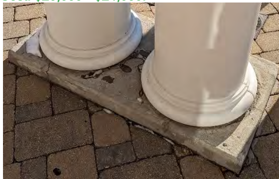
Cracked concrete at column bases.
